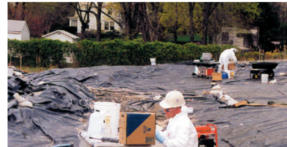
Formerly Utilized Sites Remedial Action Program. Groundwater sampling for radioactive materials, Wayne, NJ.
