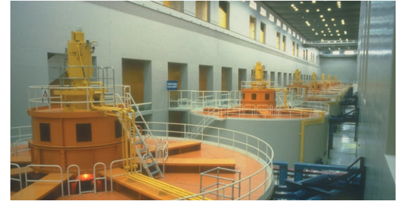
Turbines inside the Bonneville Dam powerhouse, Oregon.
