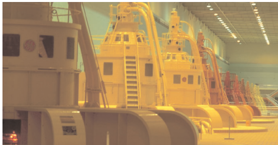
Turbines inside The Dalles Dam Powerhouse, OR.
