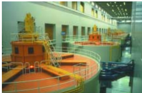
Turbines inside the Bonneville Dam powerhouse, Oregon.
