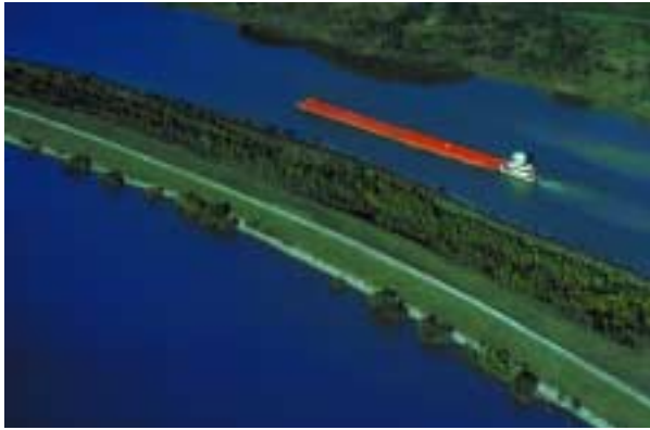
Construction is underway on the channel leading to Victoria, Texas, from the Gulf Intercoastal Waterway. The size will become the same as that of the waterway, 12 feet deep by 150 feet wide.
