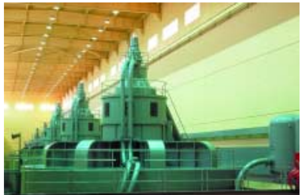
View of Ice Harbor Lock and Dam turbines.
