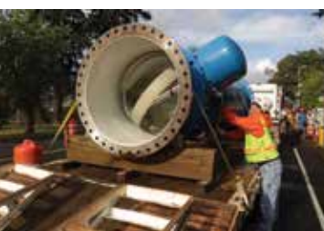
Portland, Oregon has just become the latest city to harness its water pipeline flow to produce hydroelectric power.
