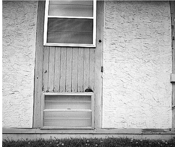
Signs of wear on exterior wood siding
