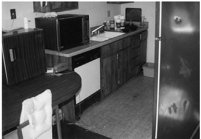
amaged floor and appliances in a kitchen awaiting renovation
