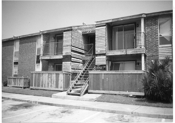
Rotten wood removed, awaiting replacement and painting
