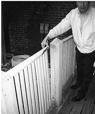
roken wooden railing on back porch of first-floor unit
