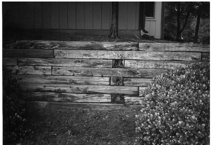
Rotten railroad ties in retaining wall
