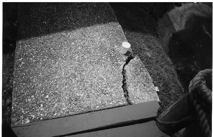
A broken sidewalk
