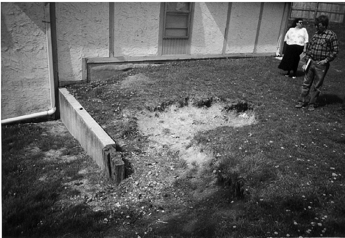
uncorrected erosion problem
