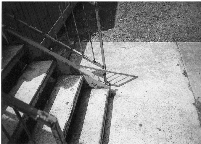
Rusted balcony railing awaiting replacement
