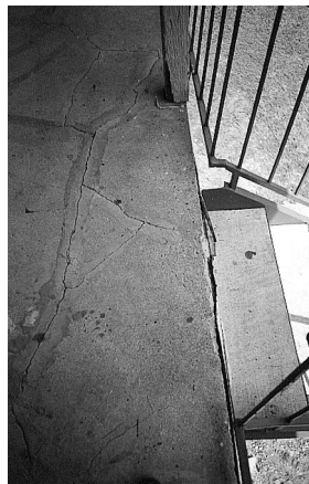
Cracked concrete and damaged frame in second floor balcony area
