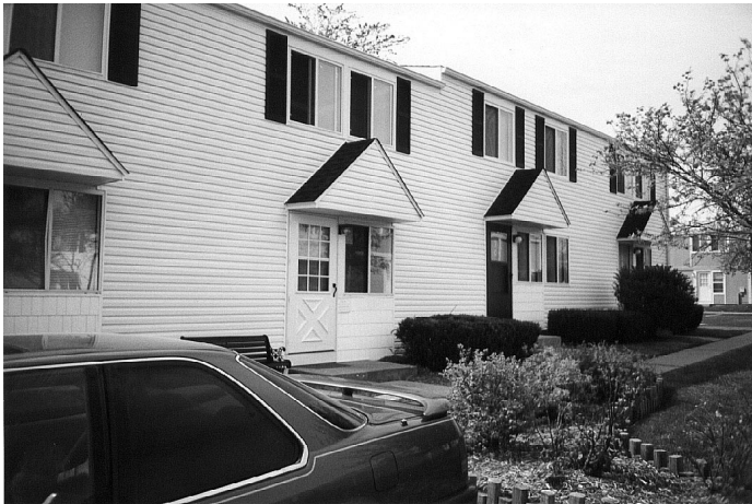
New vinyl siding, windows, and dormers for buildings at the property's entrance
