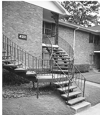
Step repair: cracked concrete covered with nonskid steel cap
