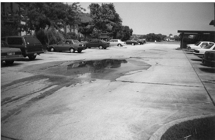
Sink hole in parking area, out for repair bids
